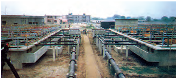
Fig. 6.7: Sewage Treatment plant under Yamuna action plan at Faridabad
